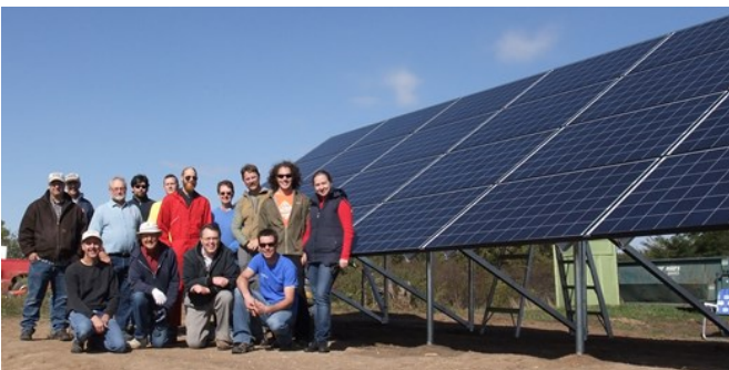
Left: Sept 2015 workshop installed a 6.24 kW Solar PV array
