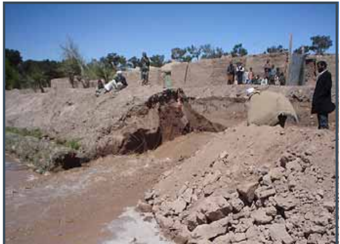
Illustration 7: Breach in main canal (April 2005)
